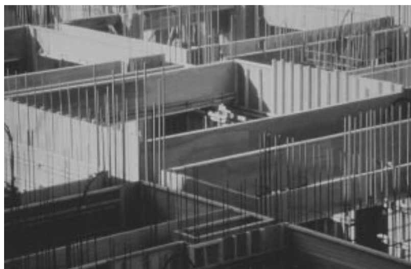
Formwork boards in Japan are made from tropical wood and are usually discarded after their initial use.
